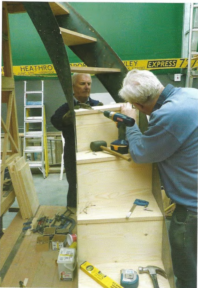
Graham Burnell and John Hutchinson working on the tricky job of constructing an NS staircase. (MHCb)
