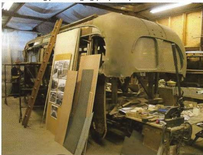
The temporary internal supporting structure of timber beams may be seen within the body of the 1929 AEC Reliance (RU8806) restoration project.
