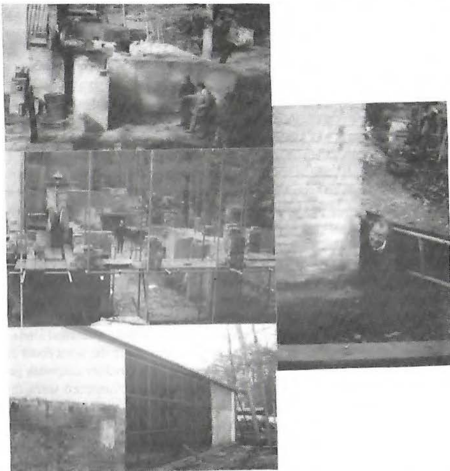
From top: 15 October 1994 , the two former shelters can be seen with roofs already removed; 22 October 1994 : Blackie Blackburn demonstrates the cavity dug for underpinning; 12 November 1994 : brickwork progressing nicely; 5 February 1995 : extensive side elevation complete. The extension will also house the towbus in 'call out' mode.
