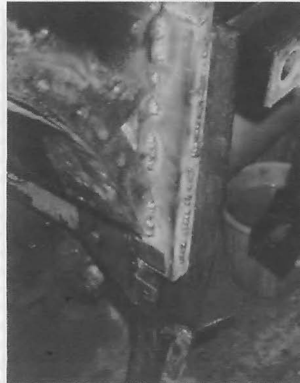
At the side, the steel box section stub was almost totally replaced. The small piece protruding over the bottom of the stub area was all that remained of the wheelarch hoop!
