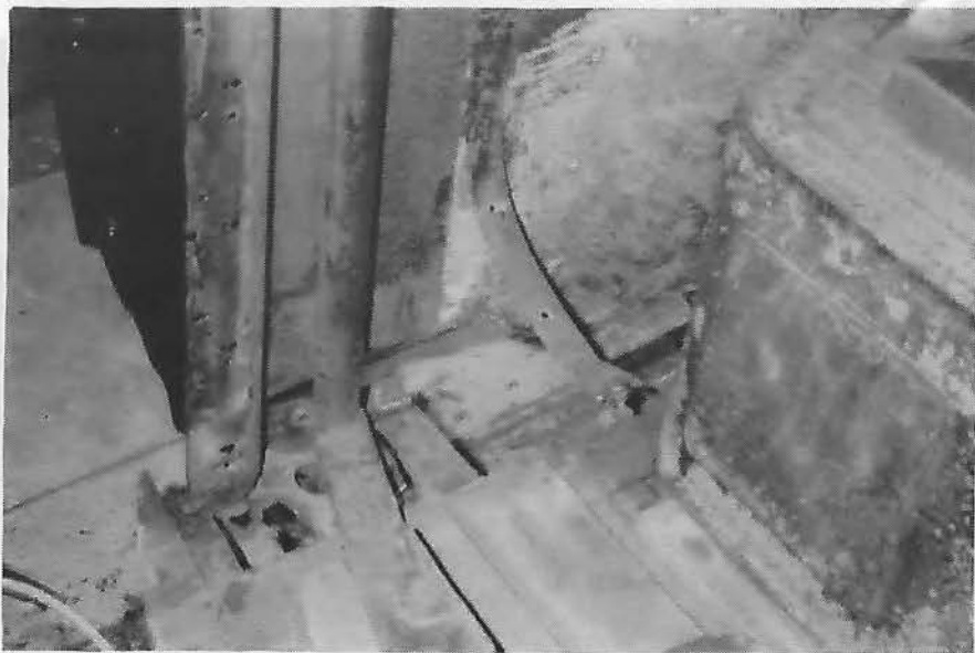
The front step area displays substantial corrosion. Note the holes by the door pivot
