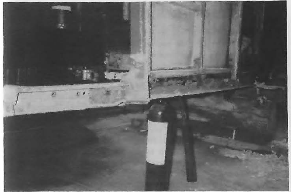
The badly rusted back rail had been previously repaired using an incorrect section.
