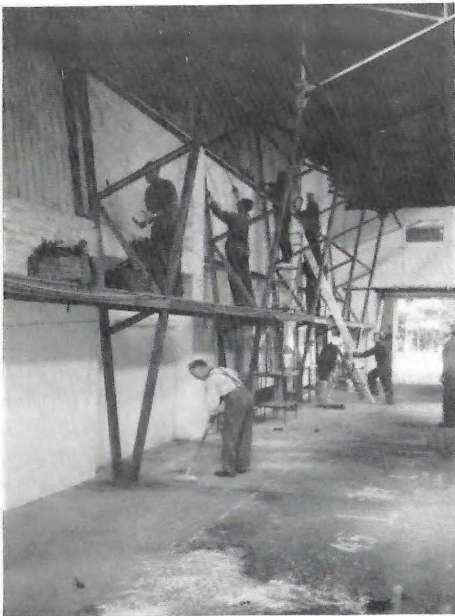
A Fresh Coat: Substantial progress was made by a dedicated team during the clear-up weekends in which 25+ years of decay was removed and a fresh coat of paint applied to the interior of the Redhill Road side of the building. It really does look brighter now when you walk in. (Photo: Colin Shepperd)
