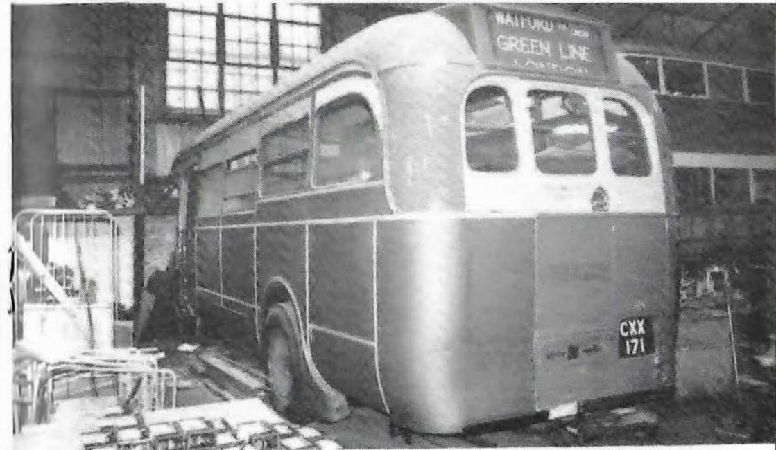
Better than new: The coachbuilding team, led by our Chairman, really are doing a magnificent job with T448, as can be seen by the quality fit of these new panels and beading. It is certainly looking healthier than T404! (Photo: Mike Nash)
