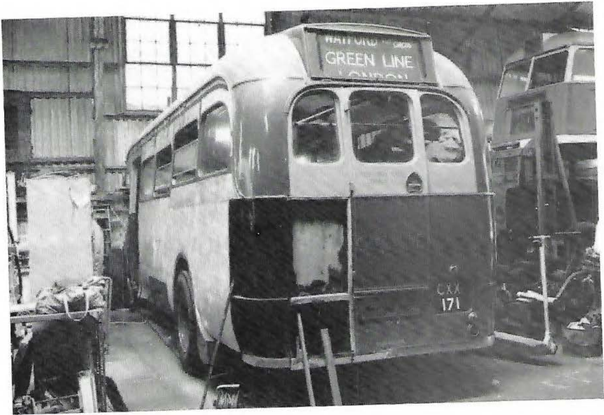
Work to the nearside of T448 is continuing at some pace thanks to many long hours put in mainly by your Chairman and Brian Down. (Photo: Mike Nash)
